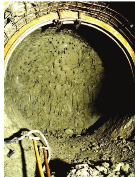
Figure 3. Circular adit used in backanalyses of the earth pressure coefficient at rest K_0 (Pavlik et al., 2004).
