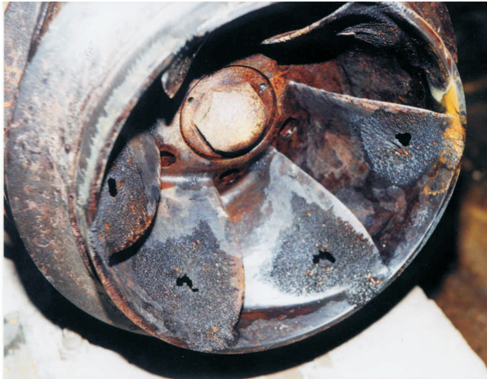
Figure 1.1: Photograph of pump damage caused by cavitation erosion[4]. Courtesy of Sigma Lutín
