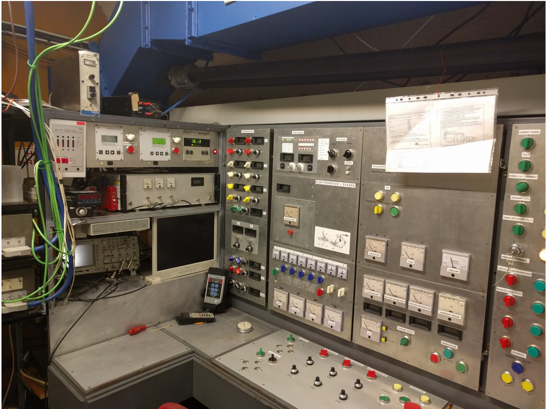
Figure 4.6: Microtron control panel
