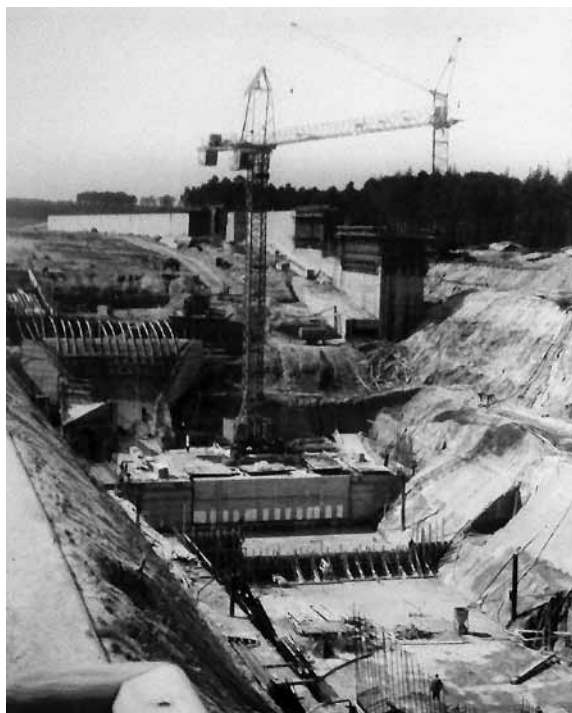
Figure 4.8 – In 1968, Czechoslovak engineers made a series of study trips to West Germany, the Netherlands, and the USSR. The experience in Germany influenced them most. This picture, taken during the trip to the RMD construction site, shows the water saving basins of the RMD lock at Erlangen. Source: Zpráva ze studijní cesty do NSR a Holandska k ekonomickým problémům vnitrozemské plavby (AVUV) [Year 1968].
