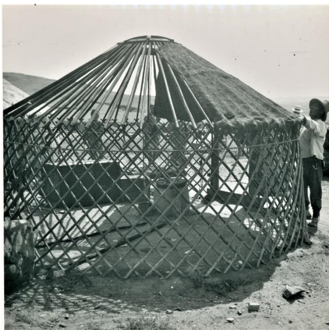
Fig. 46. A photograph of a ger under construction: the top of the trellis wall can be seen. Courtesy of the National Museum of Denmark.
